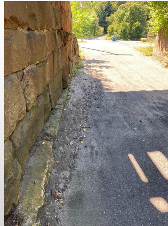
Sediment settled under RR bridge on Arch Street
