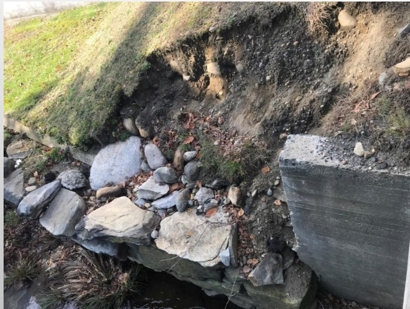
Erosion around Route 2 Bridge, 2021
