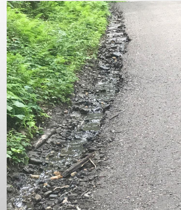
Erosion of gravel road (not in Erving/Northfield)
