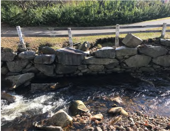
Figure 4a: Bank and wall erosion adjacent to Hanson Court, facing east
