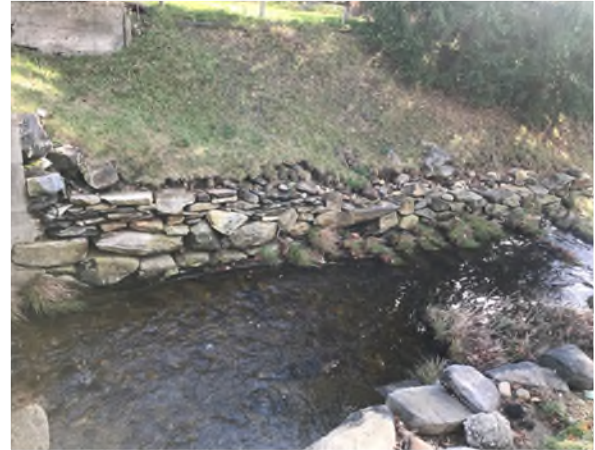
Figure 4b: Bank erosion downstream side of Route 2 bridge, east bank
