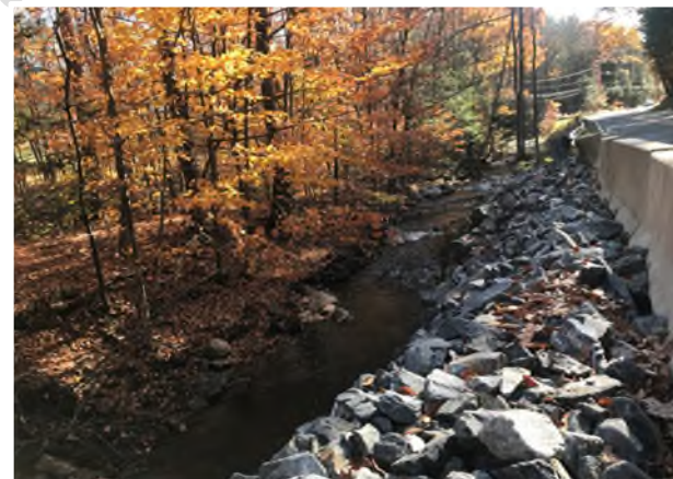
Figure 4f: Riprap placed along North Street after extensive damage to road shoulder, in which bank erosion came within three feet of a sewer main; the former Swamp Road bridge abutments are in the photo background
