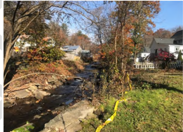
Figure 4d: Bank erosion in lower left corner at Church Street residence, facing north; note the hole in the lawn behind the retaining wall
