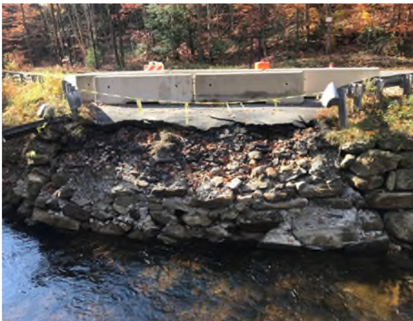
Figure 4e: Swamp Road bridge removed after structural damage, west bank
