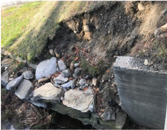
Figure 4c: Bank and wall erosion downstream side of Route 2 bridge, W bank
