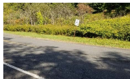
Image 12: Faded double-yellow centerline along Route 2 near MM 62.
