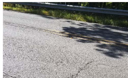
Image 15: Faded double-yellow centerline along Route 2 East of Mountain Road
