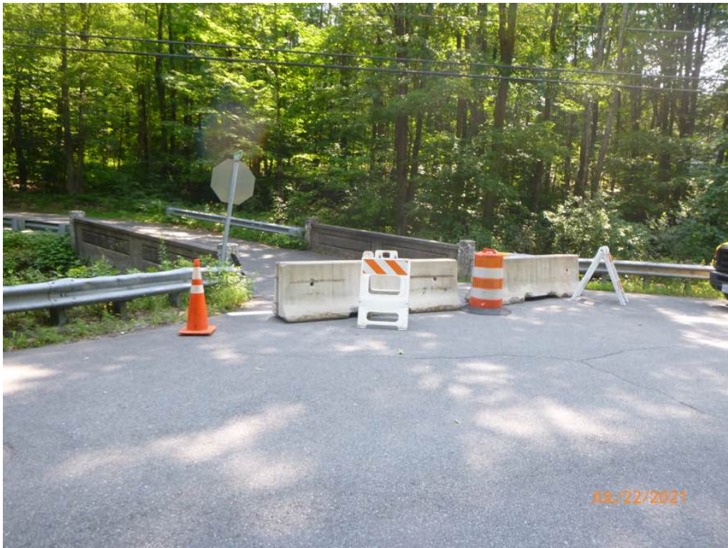
Photo 2: West of the structure, jersey barrier with reflective stands, drum, and cone are in place at the intersection of Swamp Road and North Street.
