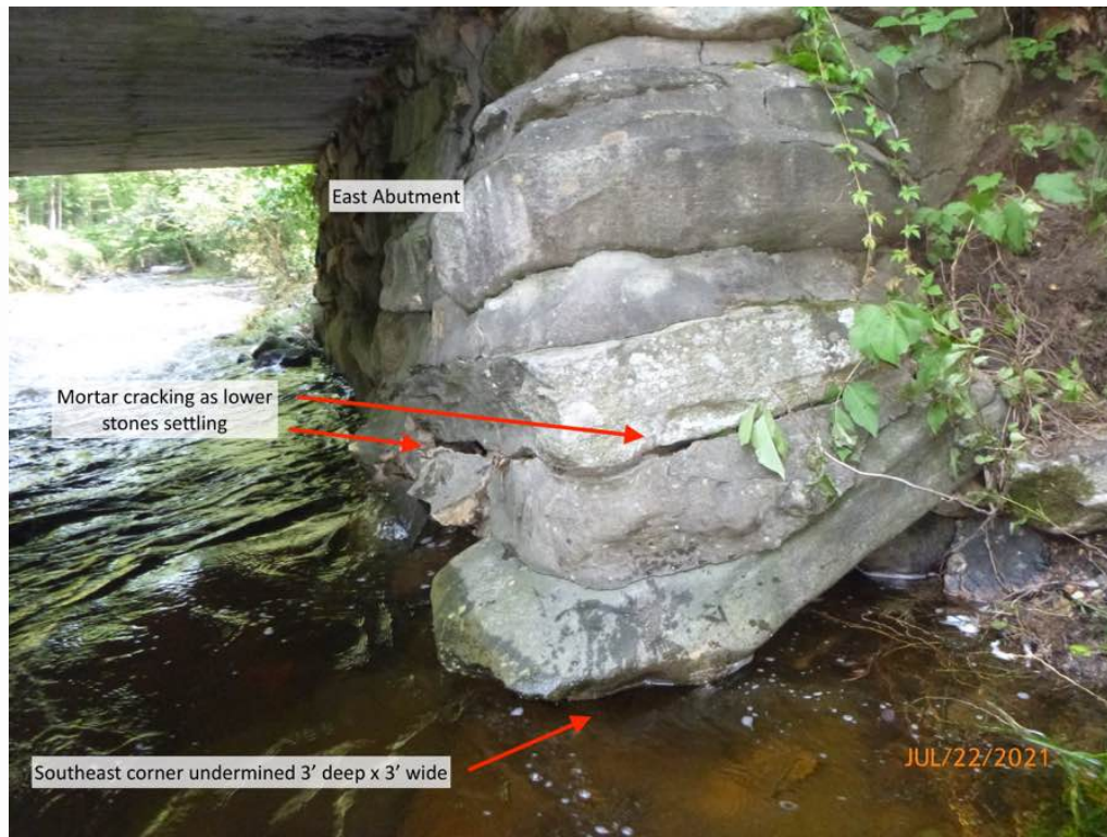
Photo 9: East Breastwall, south end has severe undermining. Lower stones are settling, which is opening gaps between stones and cracking mortar.
