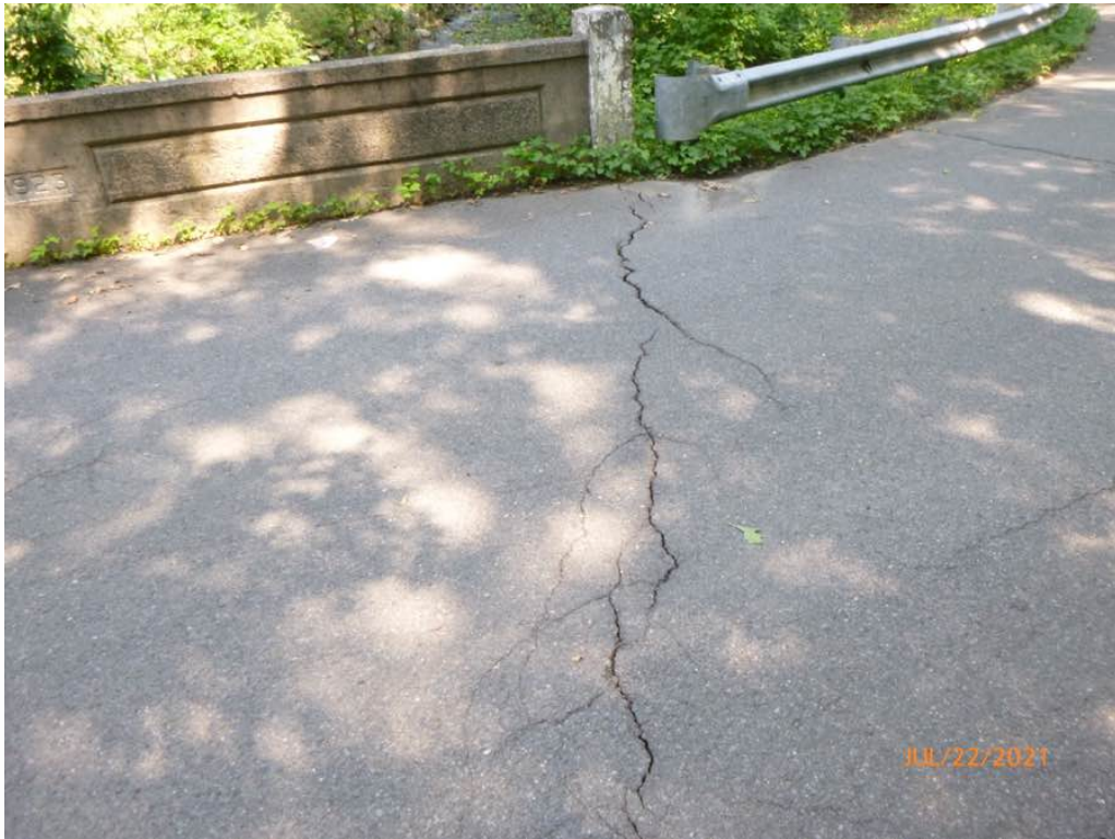
Photo 5: East Approach has transverse cracking in the roadway at the east deck end up to 1/2" wide.
