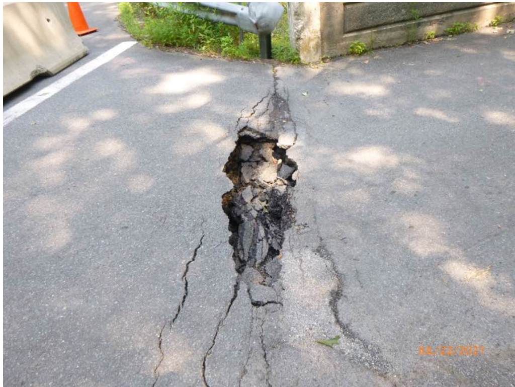
Photo 4: West Approach has a large hole in the roadway at the west deck end.
