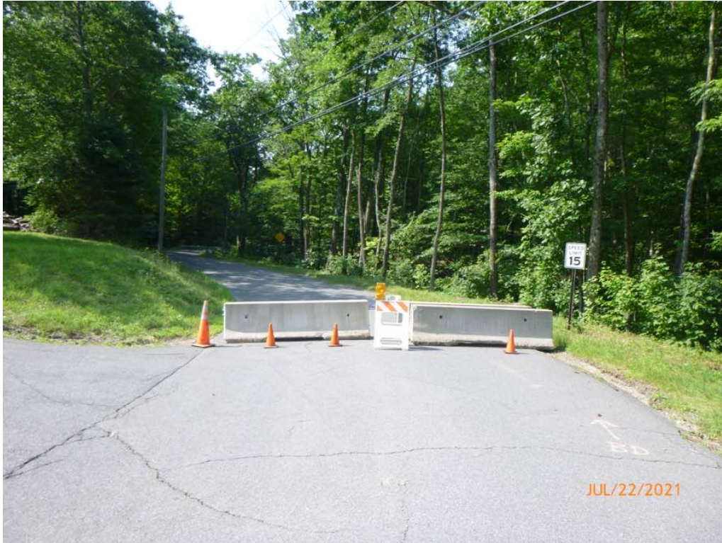
Photo 1: East of the structure, jersey barrier with reflective stand and cones are in place at the intersection of Swamp Road and High Street.
