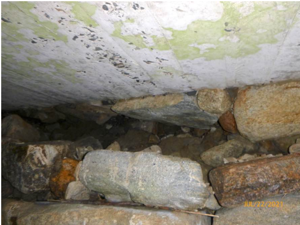
Photo 8: West Breastwall, void at the top up to 18" high x up to 3' deep.
