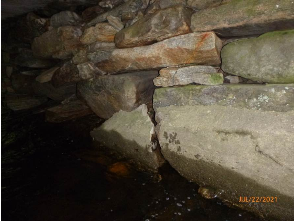
Photo 7: West Breastwall, north end concrete slab is cracked through and settled.
