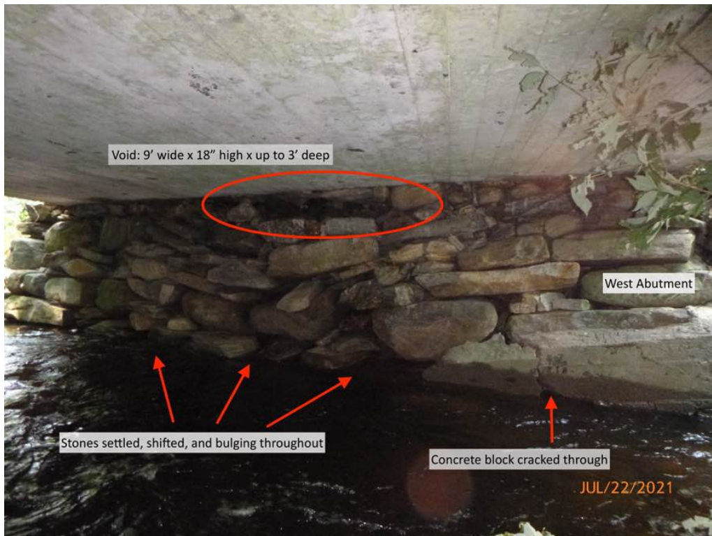
Photo 6: West Breastwall has shifted, settled, & bulging stones, many voids including a large void at the top, and a cracked concrete slab at the north end.
