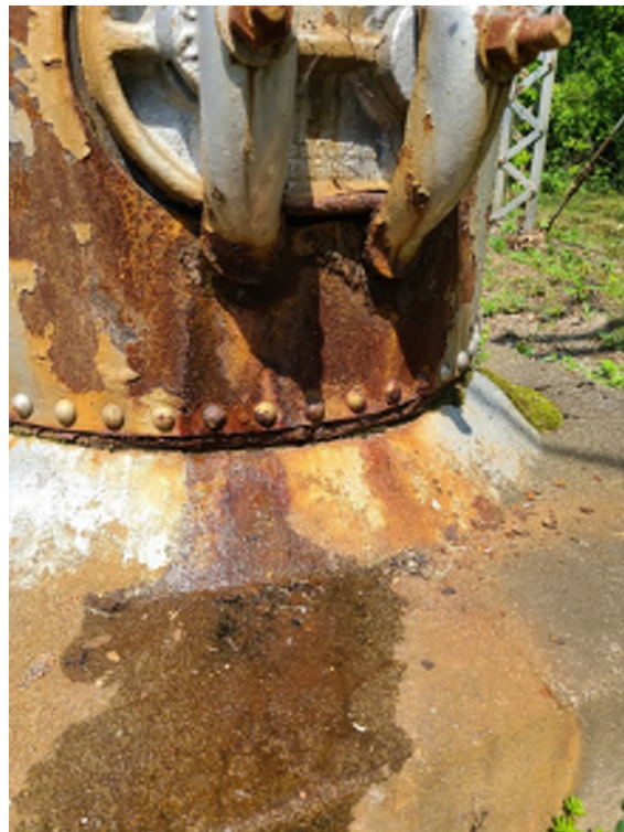
Photo 7: Water leak at base of water column, minor steel corrosion from leak
