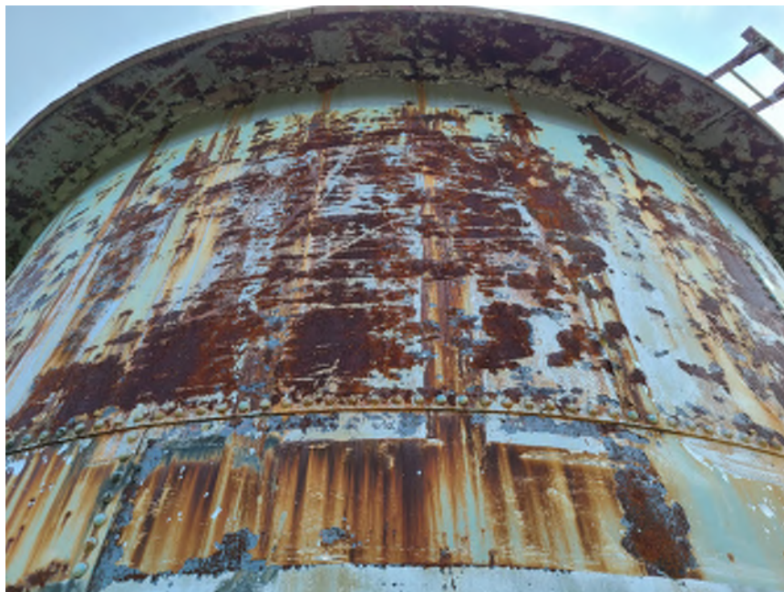
Photo 5: Typical tank surface condition, note cleaner steel where flaking paint had been collected
